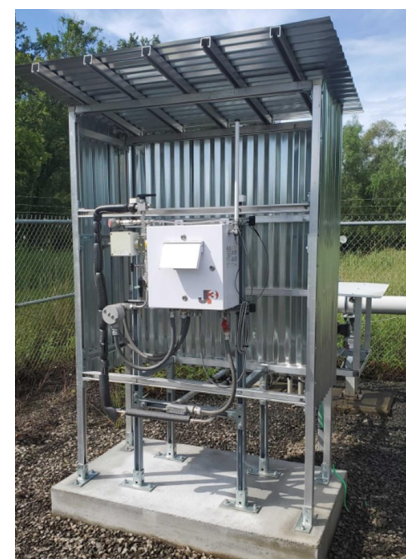
Verax SSL Installation
